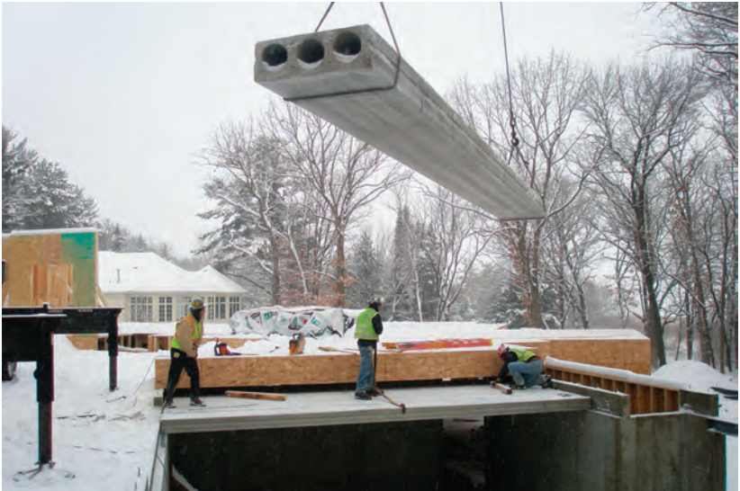
FIGURE 2-6 Precast concrete is outside the prescriptive provisions of the MRC but is approved as an engineered system and inspected for conformance to the construction documents.
