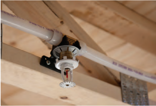
FIGURE 9-1 Residential sprinkler in multipurpose loop system using PEX tubing (Courtesy of Uponor Inc.)
