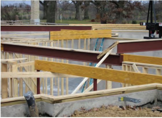
FIGURE 4-1 Concrete, dimension lumber, engineered wood and steel structural elements of a single-family dwelling
